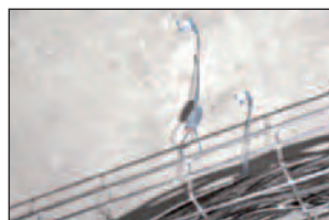
Light weight Cable Trays / Lights
