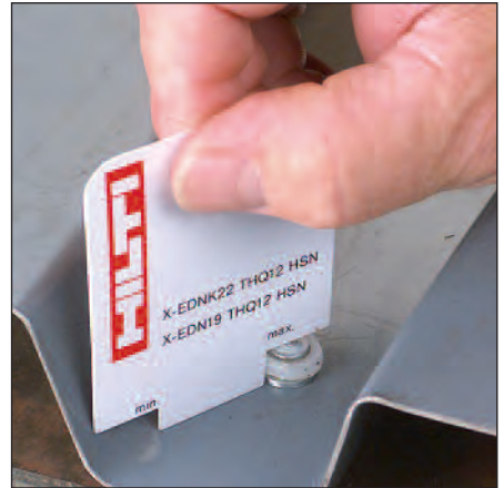
Checking the standoff of an X-EDN 19 roof deck fastening with a plastic template
