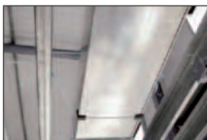
Square Air Ducts
